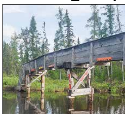
Left: An above-ground portion of the Ely water line from Burnside Lake, which was built in 1932.
