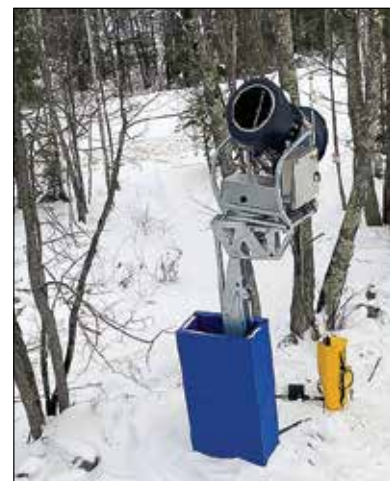
Giants Ridge has added 74 new snowmaking machines, significantly improving the facility's ability to create artificial snow.
