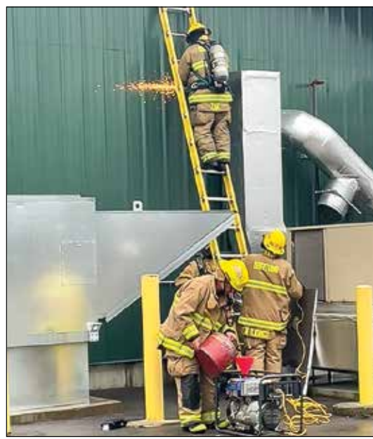
Sparks fly as firefighters used metal saws and grinders to cut through metal sheathing to expose and extinguish fire at Lamppa Manufacturing.
