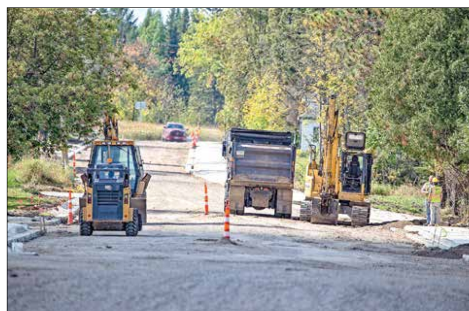
Top: Construction workers put down a second layer of asphalt on the westbound land of Hwy 115 east of Cook on Tuesday. The resurfacing of the highway from Cook to Peyla has been done in two stages and is nearing completion.
