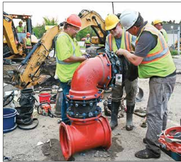
Workers assemble one of the critical junctions above ground before lowering into position underground. photo by C. Clark
