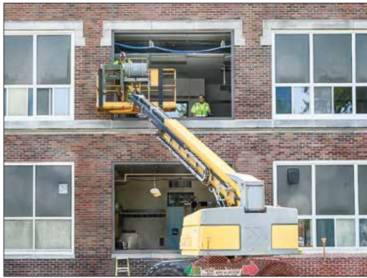
Gaping holes in the front of Ely Memorial High School as workers continue to install windows at the school at 8:15 a.m. on the first day of school on Tuesday. photo by C. Clark
