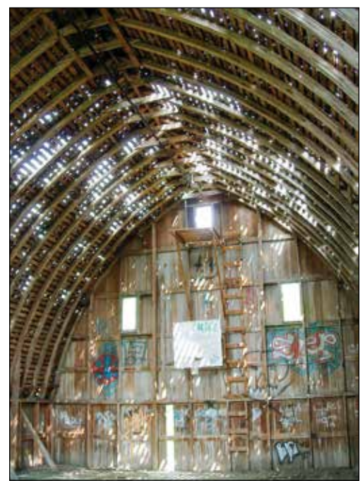
Above: The barn in a 2005 photo showing the extensive roof damage and also the basketball hoop used by local youths for pickup games.
