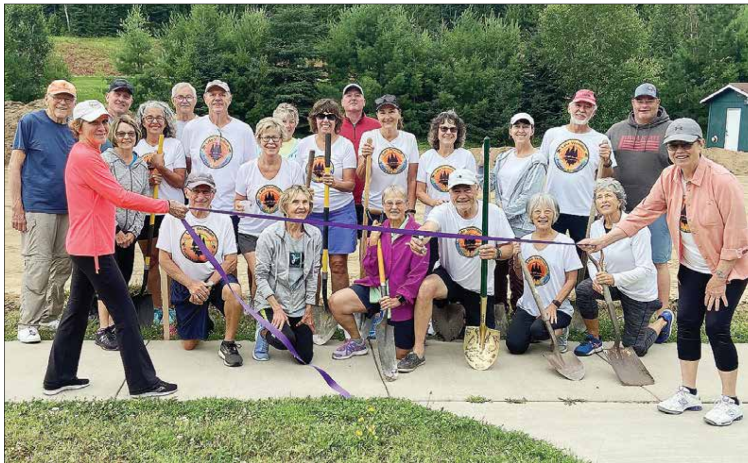
GREENWOOD TWP- Lake Vermilion Pickleball Association members gathered Tuesday to watch as construction began on the new pickleball courts at Greenwood Town Hall. The four-court area is expected to be paved by Aug. 1, with fencing installed sometime in August. The courts are being installed adjacent to the pavilion, bocce ball, and playground area. The grounds at the town hall also include a tennis court, which can be used as two pickleball courts. The project is being funded by a $25,000 donation by the township, grant funding, and many private donations. An upcoming fundraiser is set for Aug. 22 at Tavern in the Bay from 6 - 9 p.m. Donation is $10 at the door. There will be raffles, prizes, free appetizers, and live music with the Beefeater Brothers. submitted photo
