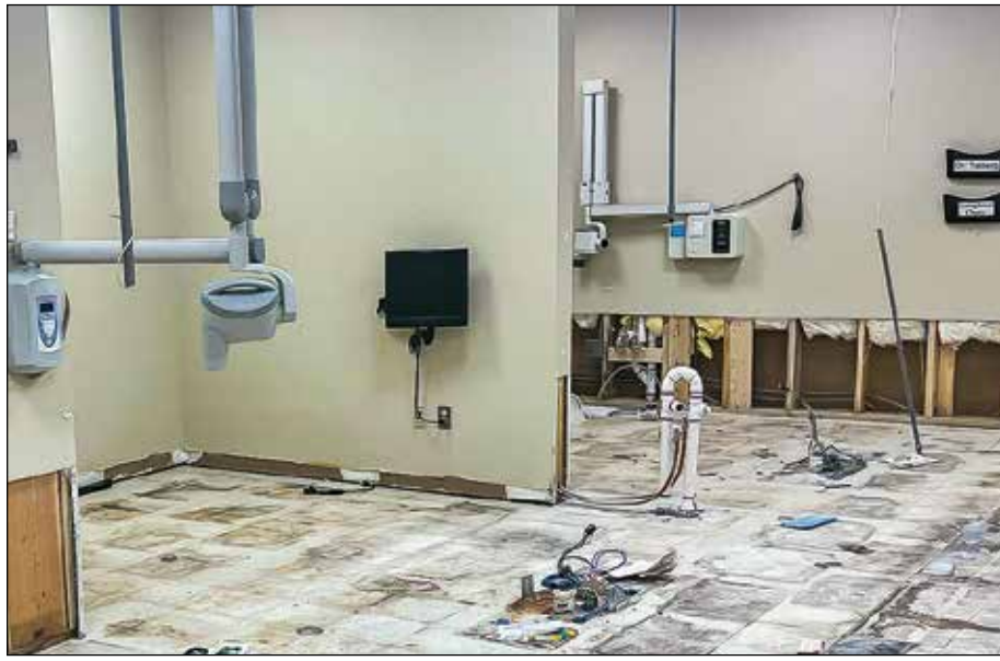
Left: Extensive wall and floor damage at Scenic Rivers Dental Clinic will be covered by flood insurance, but costly medical equipment and other contents of the building will not.
