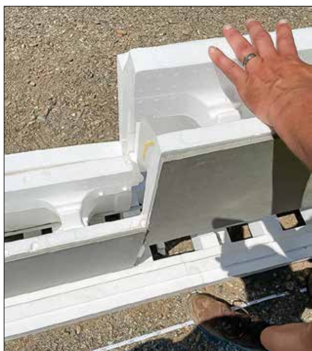
Contractor Shawn Webster slides another piece of pre-made insulating foundation form into place above the foundation footing. The forms, imported from Norway, are manufactured by Vartdal Plast, a company which is looking to enter the U.S. market. The forms interlock perfectly and come with a prefinished composite exterior requiring no further finishing. Once the forms are in place, concrete is poured and the foundation is complete once cured.
