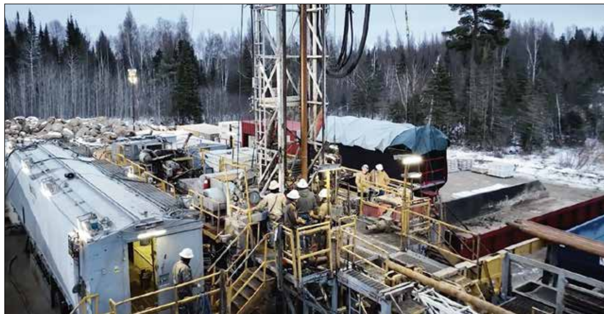
The drill rig in February at Pulsar Helium's exploratory borehole site southeast of Babbitt. submitted photo
