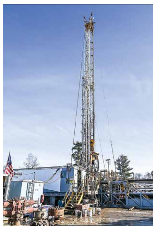
An oil and gas rig out of Wyoming is now on the Pulsar Helium site for exploratory boring.
