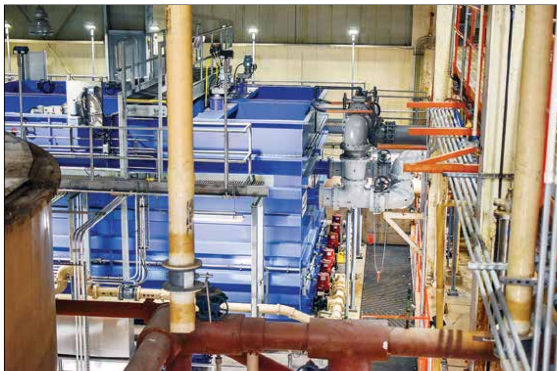
The new cloth media filtration unit at Ely's waste water treatment facility. The unit replaces an old sand filtration unit which was inadequate to meet stricter federal mercury standards. photo by C. Clark
