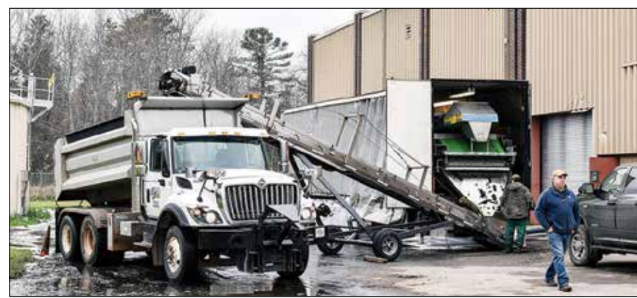
A Komline Sanderson belt press in operation on Friday, Nov. 3, at the Ely Waste Water Treatment Facility. Ely tested the unit for four days last week and achieved a six-times reduction in biosolids volume, which could save the city a lot of money in transportation costs alone. photo by C. Clark
