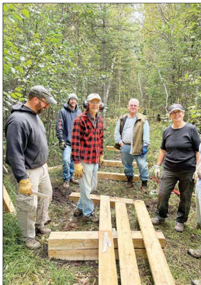
The main entrance to the trail system starts with a 500-plus foot long section of boardwalk. This new section gets hikers over a low spot that is often very wet (though it is dry at this time). submitted photos
