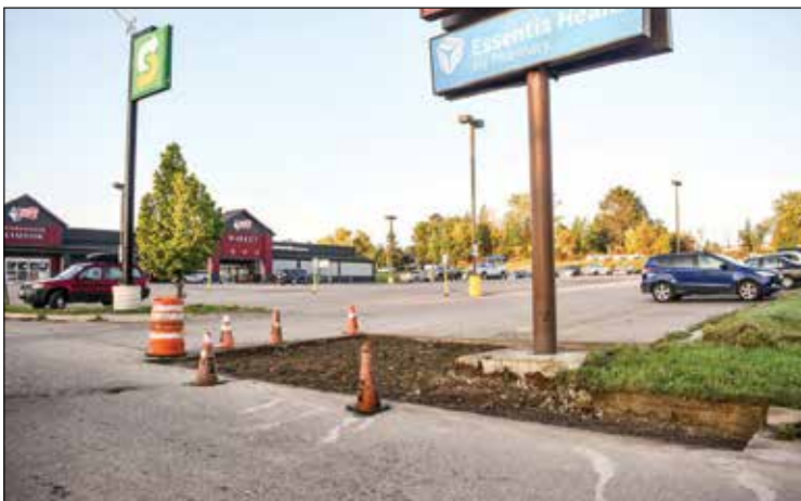
The demise of the curb and paving of Ely's worst right turn into the Zup's parking lot: the material constricting the turn has been dug out and now will be paved over. photo by C. Clark
