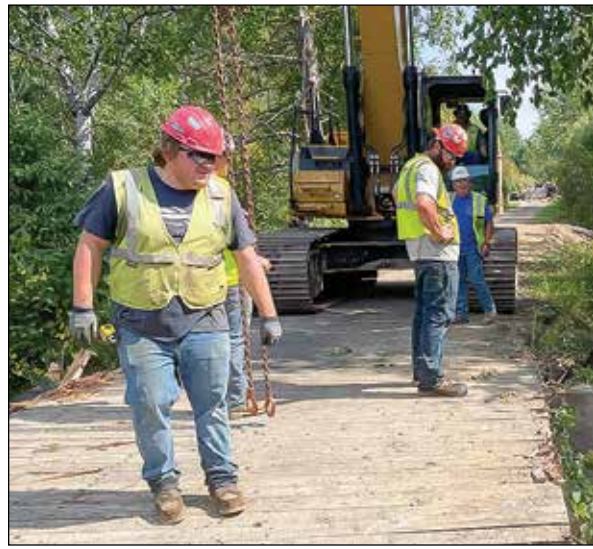
Workers were busy dismantling the dilapidated Mesabi Trail bridge over the East Two River on Tuesday. Work on the bridge should be completed by the end of the month. photo by M. HelMBERGER
