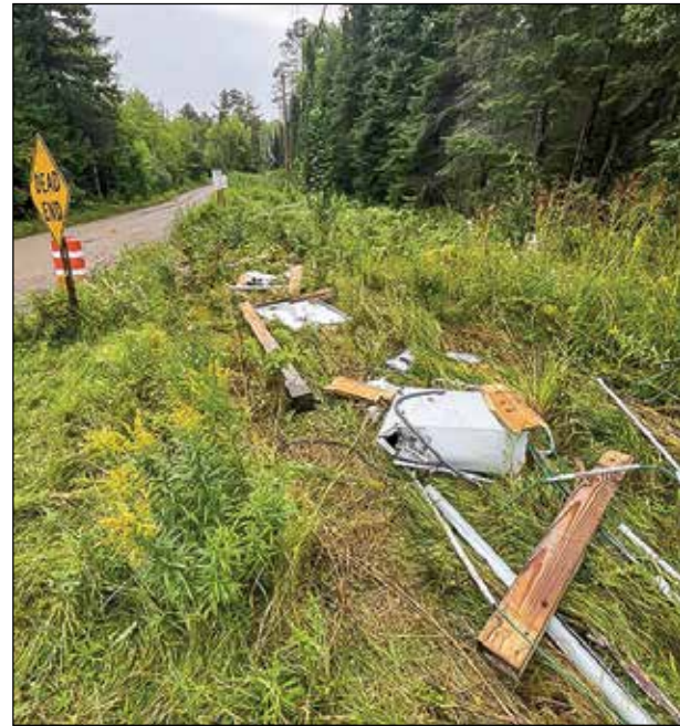
Right: The smashed Frontier phone and internet link that served McKinley Park Acres on Lake Vermilion. The service was out at least through Tuesday.
