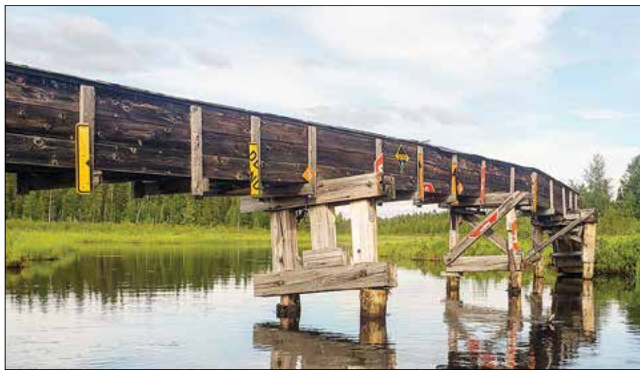
The piers supporting Ely's water intake line as they cross the open water of Burntside Lake. The structure seen here was built 1931-32. The water line updated in the 1970s is in the wooden box sitting on the top of the piers. This photo was taken during a city inspection of the intake structure during the summer of 2022. photo by Harold Langowski
