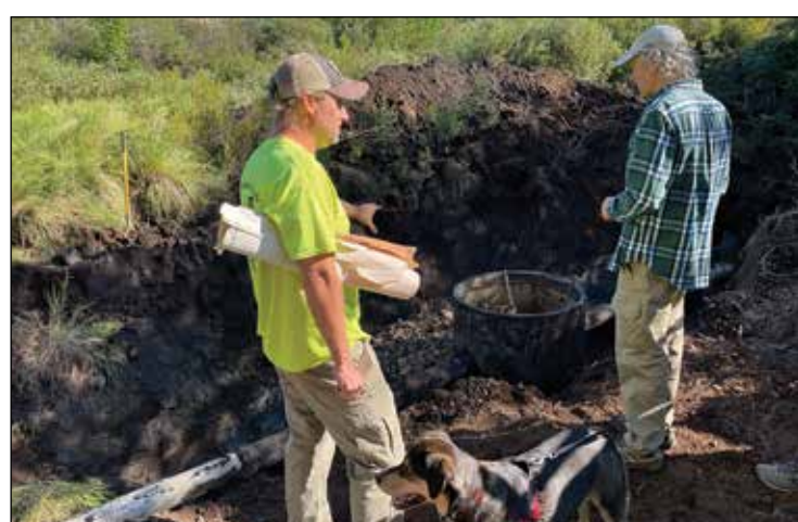
Tower-Breitung Wastewater Plant manager Matt Tichel shows work being done back in 2021 on the forced sewer main line, which runs along the Mesabi Trail in Tower. This project is still only partially completed. This manhole was replaced early because water levels were low, making it easier to work in the swampy area. photo by J. Summit
