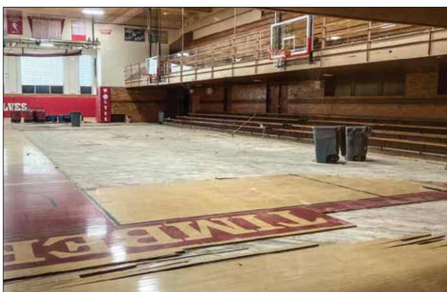
The floor of the Ely Memorial High School gymnasium where the top layer of water-damaged maple floorboards had already been removed. The floor was damaged by water from a pipe leak on March 17. photo by C. Clark
