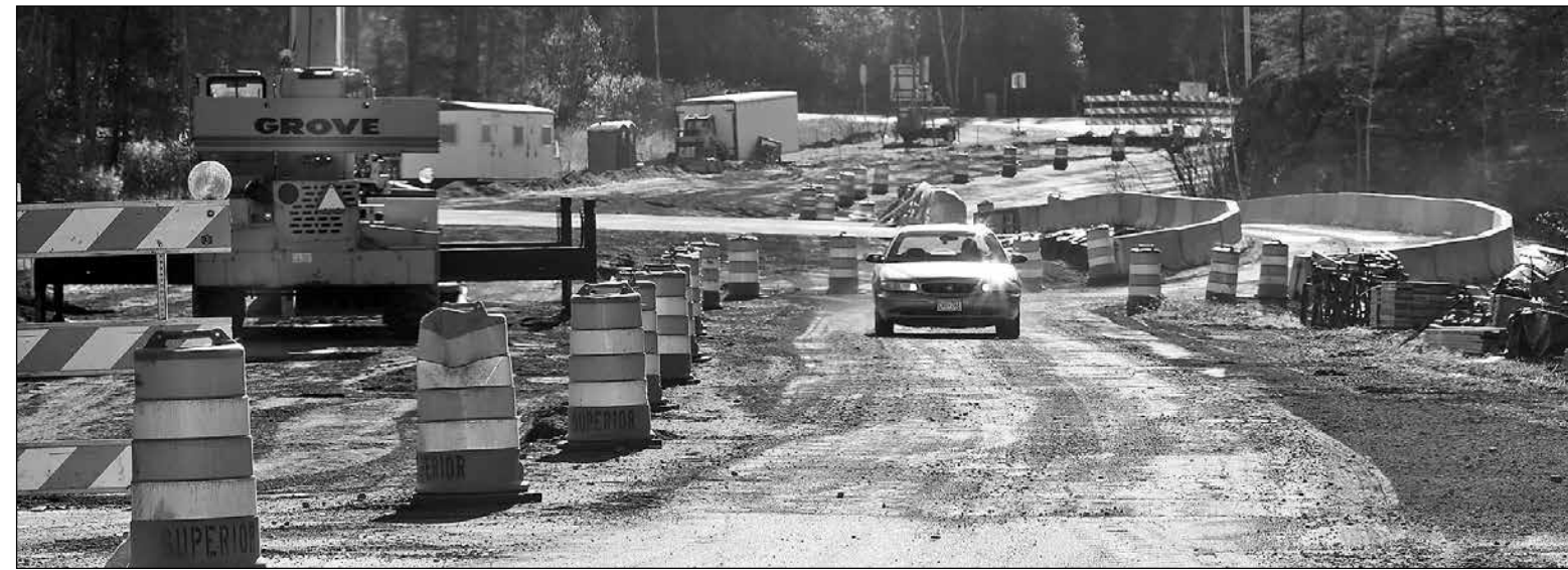
The Highway 21 bridge project between Ely and Babbitt continued this week. A one-lane drive-around access at the construction site is controlled by a traffic light for one-way traffic, avoiding a long detour. The Minnesota Department of Transportation project should wrap up this year. photo by K. Vandervort
