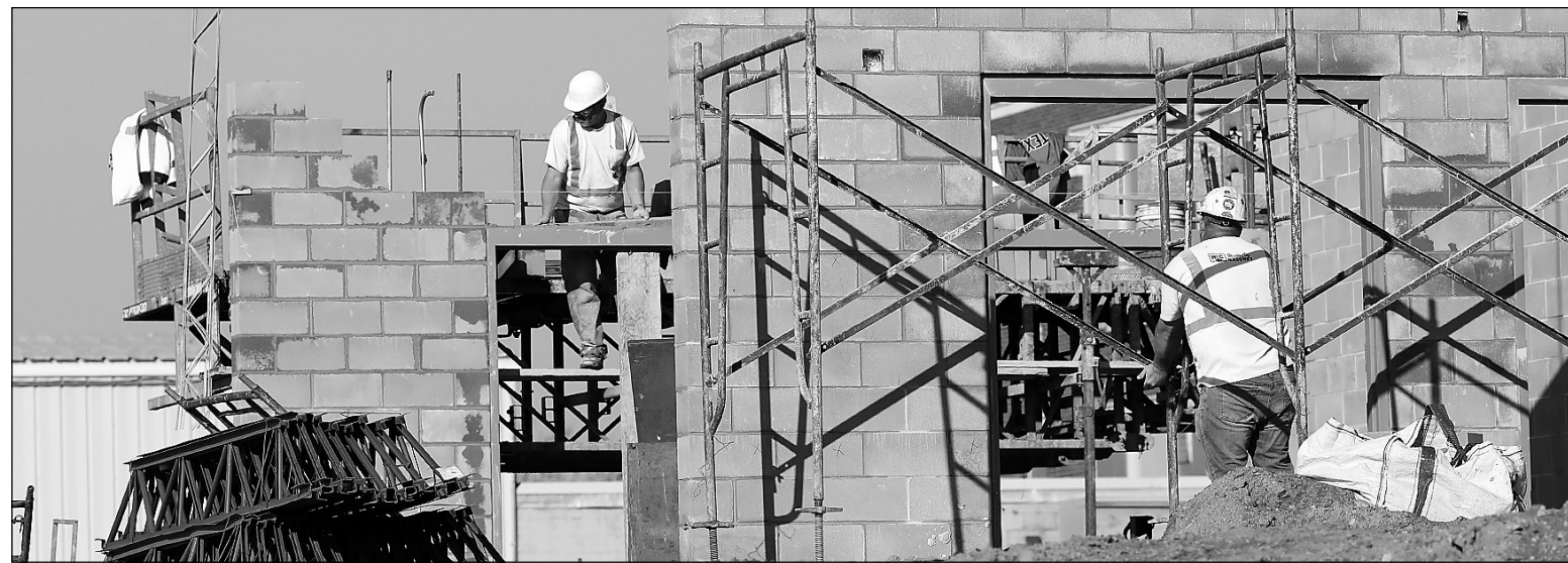
Bricklayers built interior walls Tuesday morning at the Ely School District facility renovation project. photo by K. Vandervort
