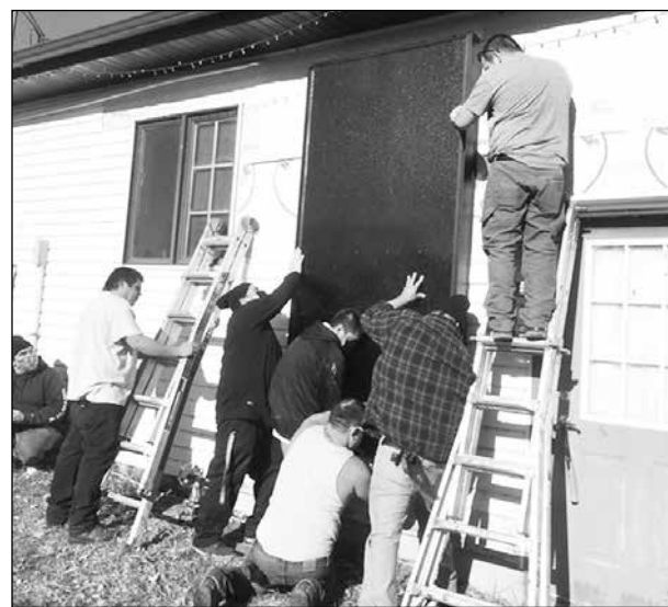
A team works to install solar panels on a Vermilion Reservation elder's home, free of charge. submitted photo
