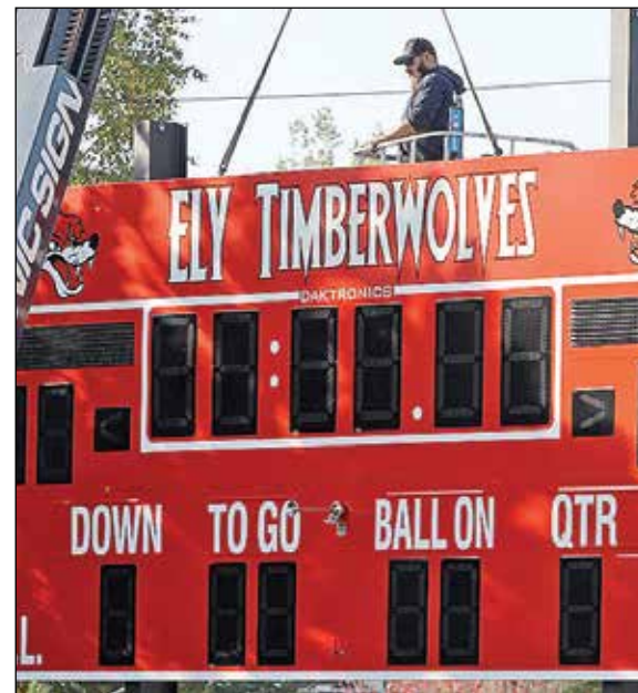
Right: A sign company worker assists with the installation of Ely's new sports scoreboard this week. photos by K. Vandervort
