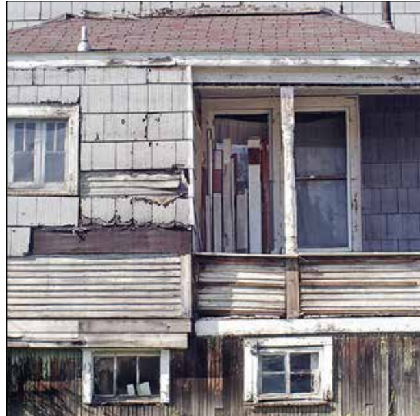
Missing siding and a generally run-down condition of an abandoned house at 106 E. Harvey St. that is owned by an Ely city council member. photo by K. Vandervort
