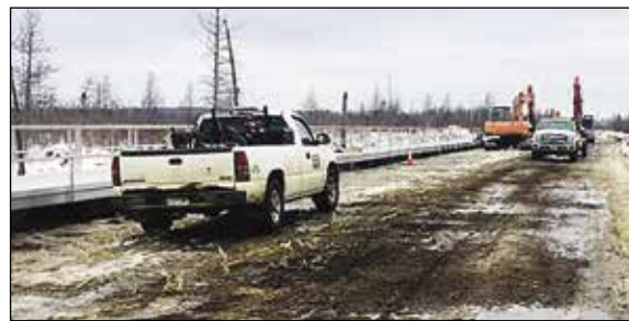
Contractors were working this week to install nearly a mile of floating boardwalk through the Darwin S. Myers Wildlife Management area in Embarrass. The work is part of the continuing effort to complete the Mesabi Trail from Grand Rapids to Ely. submitted
