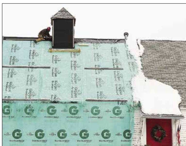
A Hammerlund Construction worker was busy enclosing a cupola at the roof peak of the Lake Vermilion Cultural Center on Monday, despite windchills of minus-35. photo by J. Summit
