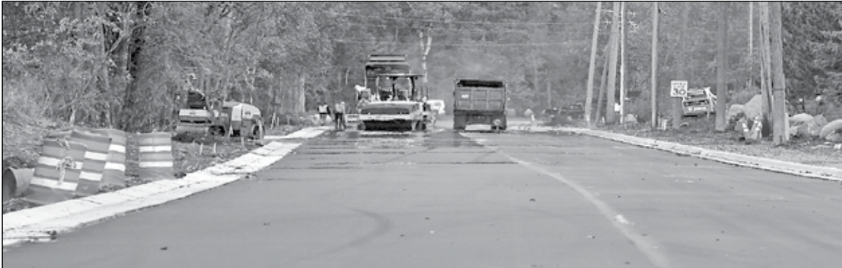
Work is nearly completed on 17th Avenue near Vermilion Community College. photo by K. Vandervort
