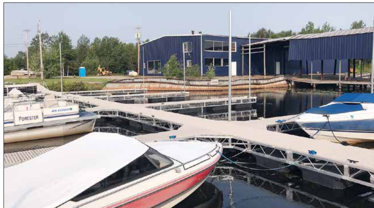
Tower's old marina, now owned by Your Boat Club and operated as a full-service marina, has new docks and slips, and renovations are underway on the marina building. photo by M. Helmberger
