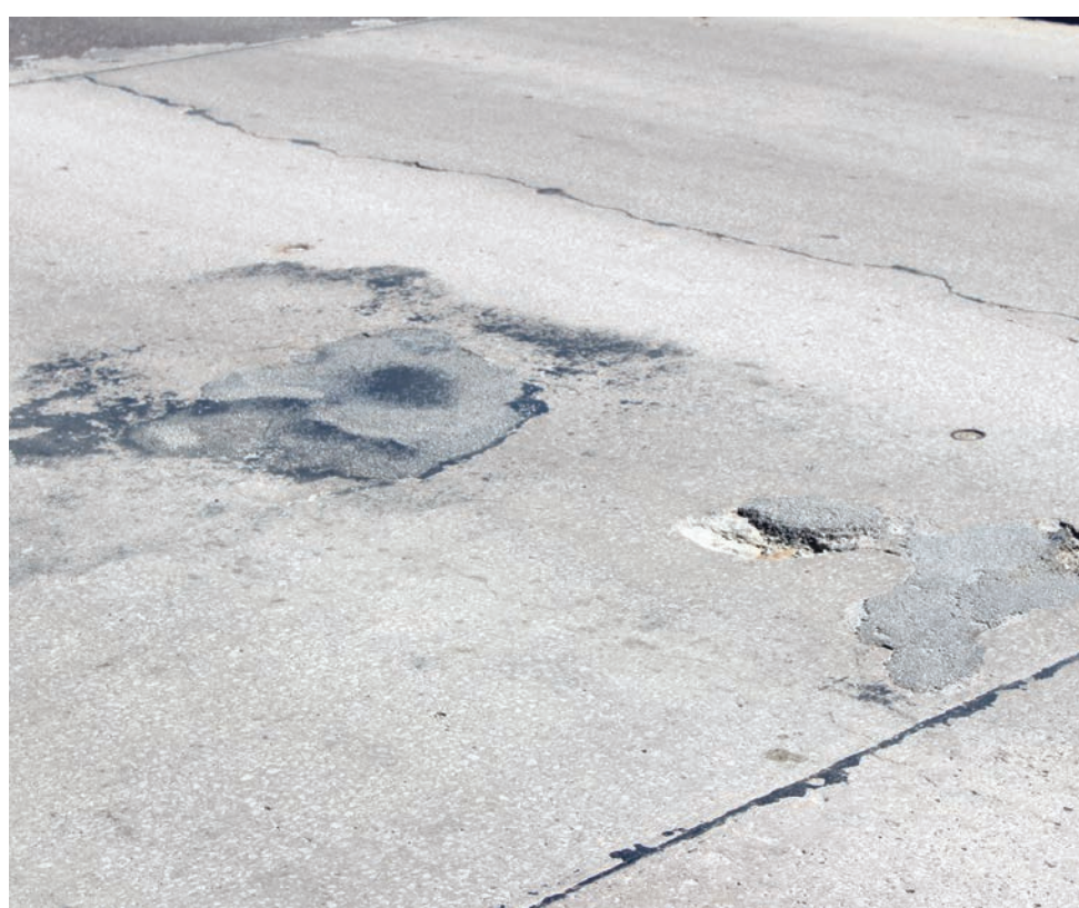
The bridge over Highway 50 contains many potholes, dilapidation, and wear across it on Wednesday, April 17, on Holden Street.
