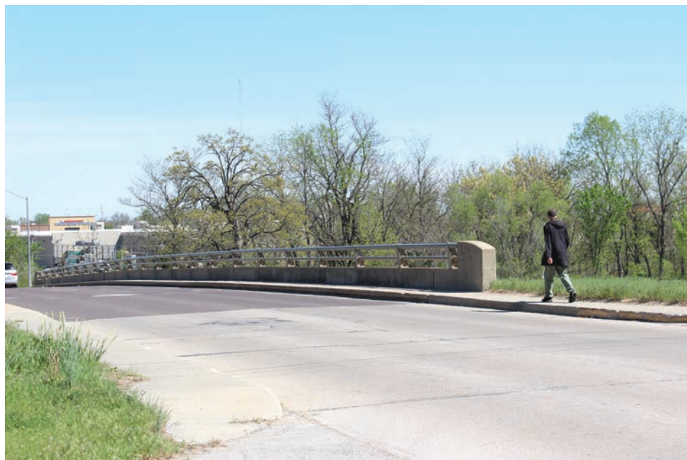
A man begins to walk on the bridge over Highway 50 on Wednesday, April 17, on Holden Street. "The major bridge over 50 is something where we are actively partnering with MoDOT to try to come together to get a plan in place to fix or replace the bridge," Warrensburg Assistant City Manager and Public Works Director Enrico Villegas said. PHOTOS BY ZACH BOTT | STAR-JOURNAL
