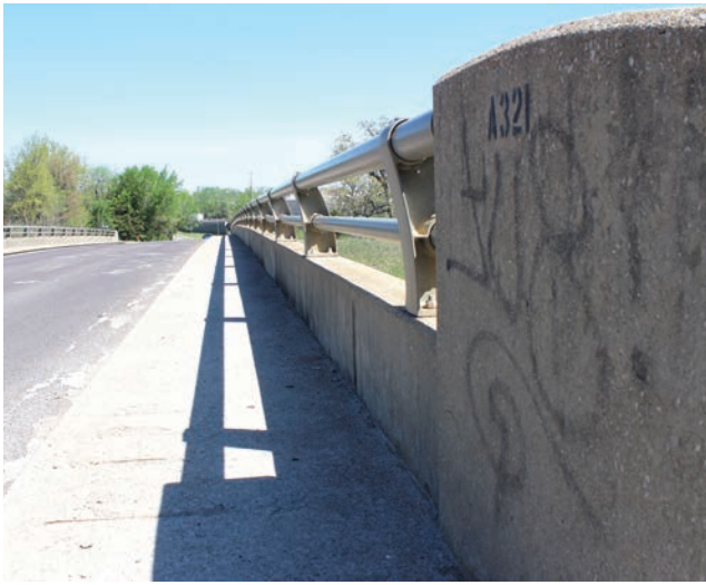
Graffiti and rubble line the bridge over Highway 50 on Wednesday, April 17, on Holden Street. The bridge is set to be improved in Phase 2 of the City of Warrensburg's Rethink Maguire project, sometime in 2025. PHOTO BY ZACH BOTT | STAR-JOURNAL
