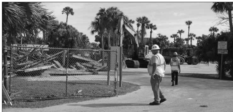
St. Johns County has contracted and granted permission to A.J. Johns Inc., a Jacksonville-based construction company, to use the parking lot to transport truckloads of sand from there to residents' homes.
