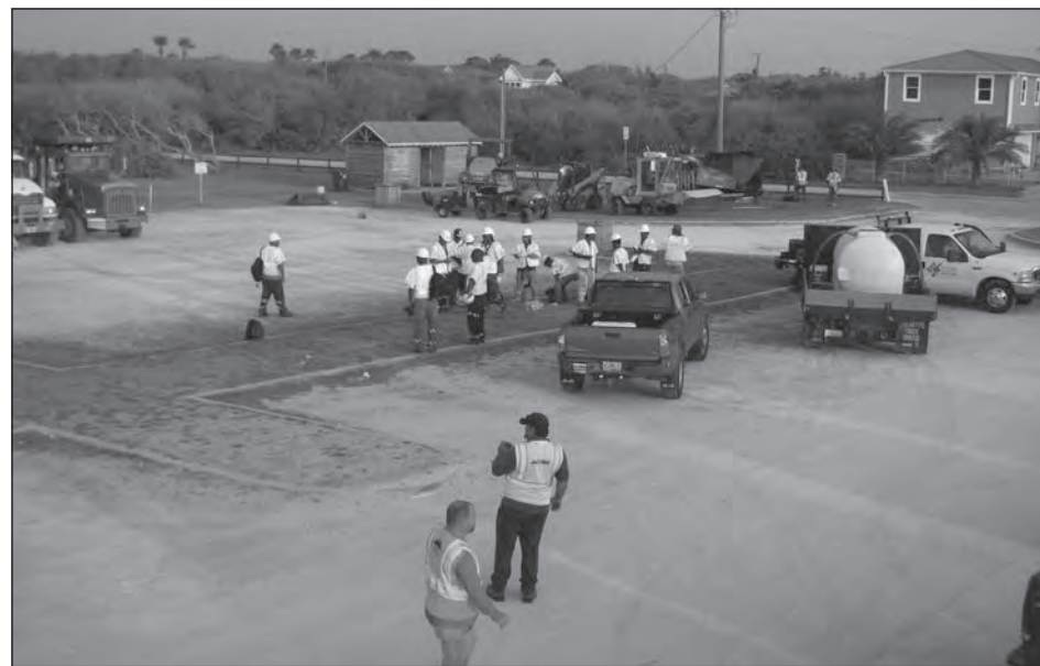
Construction to remove the A1A rumble stripes starts on the Vilano Beach end of the roadway.
