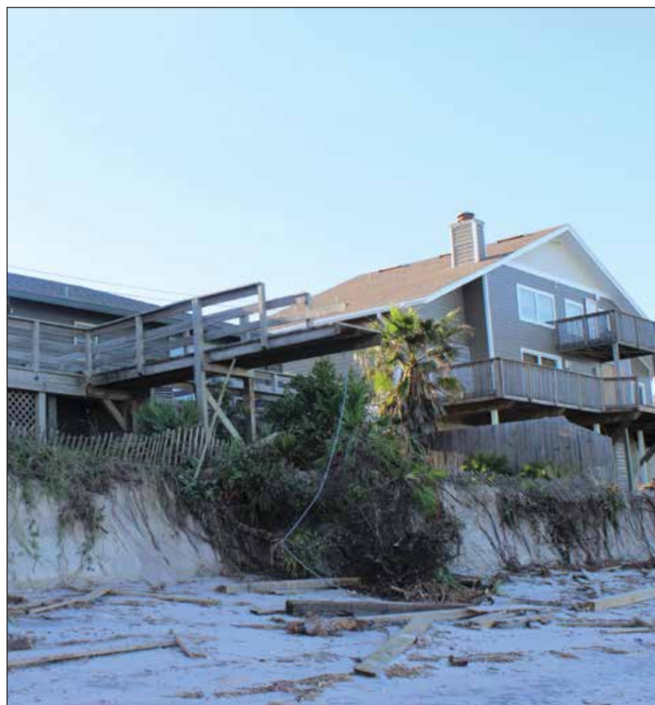
Photos by Susan Griffin A house in South Ponte Vedra Beach that sustained significant erosion as a result of Hurricane Matthew.
