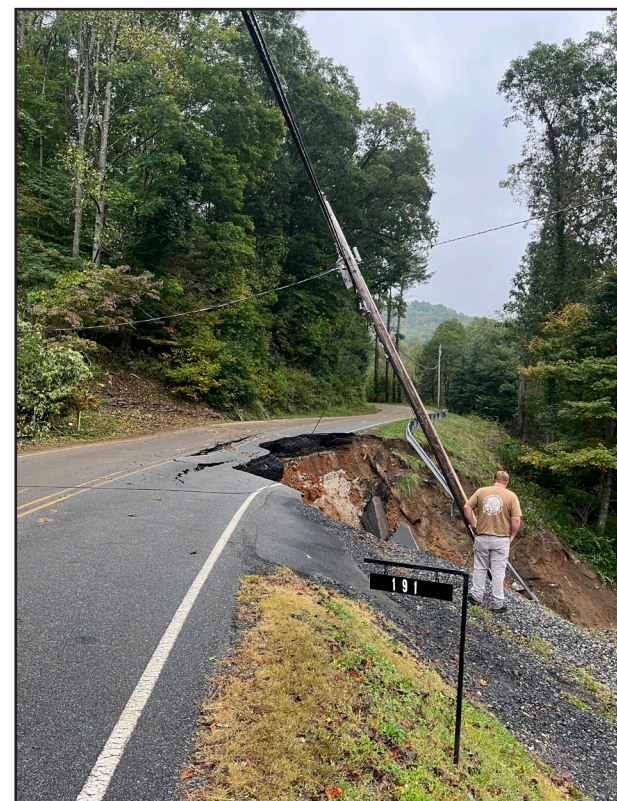
A crumbling road in Avery County, North Carolina
