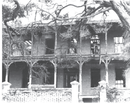
The Keeper's House in disrepair.
