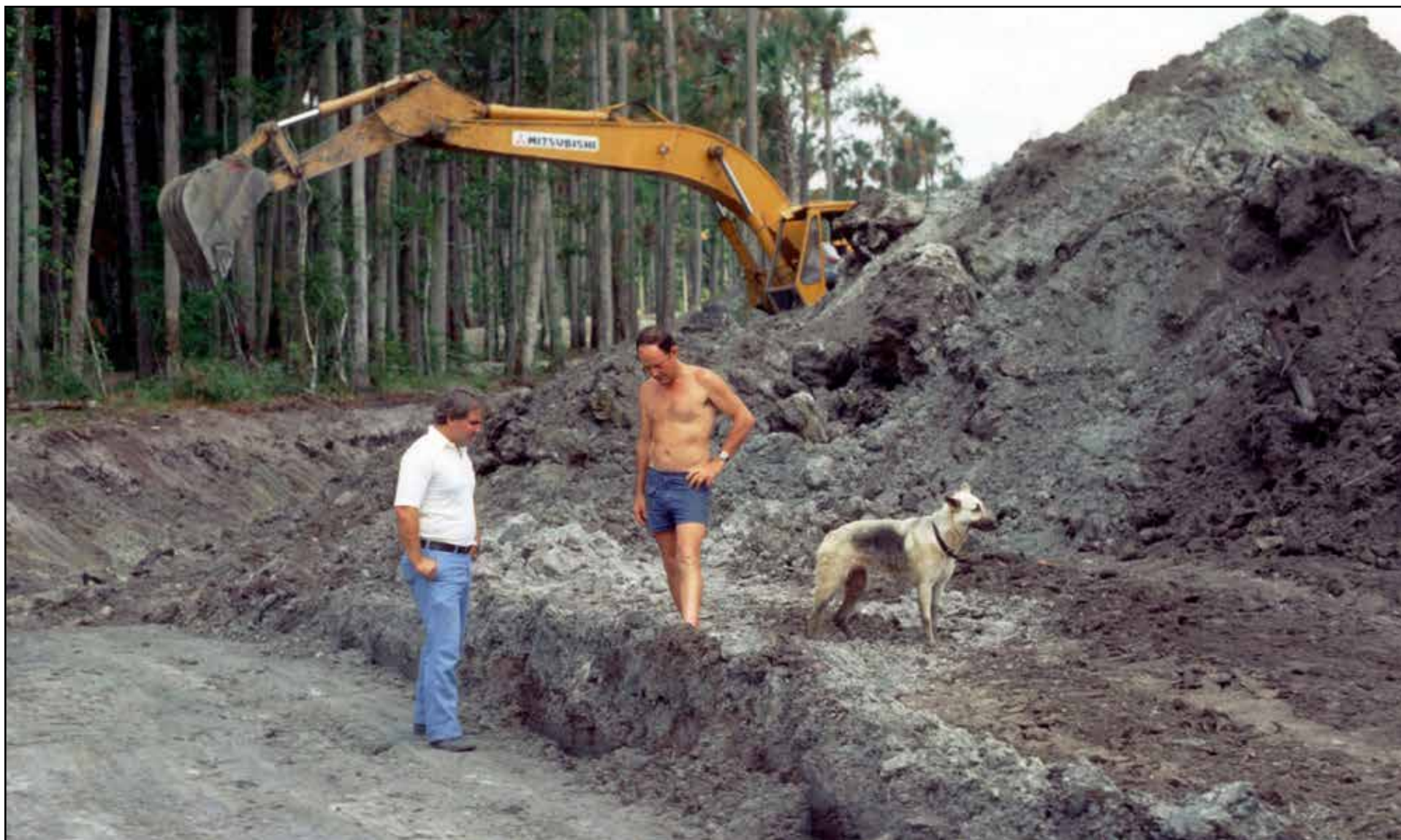
Pete Dye (right) and project manager Vernon Kelly overlook the construction of the iconic TPC Sawgrass course 40 years ago.
