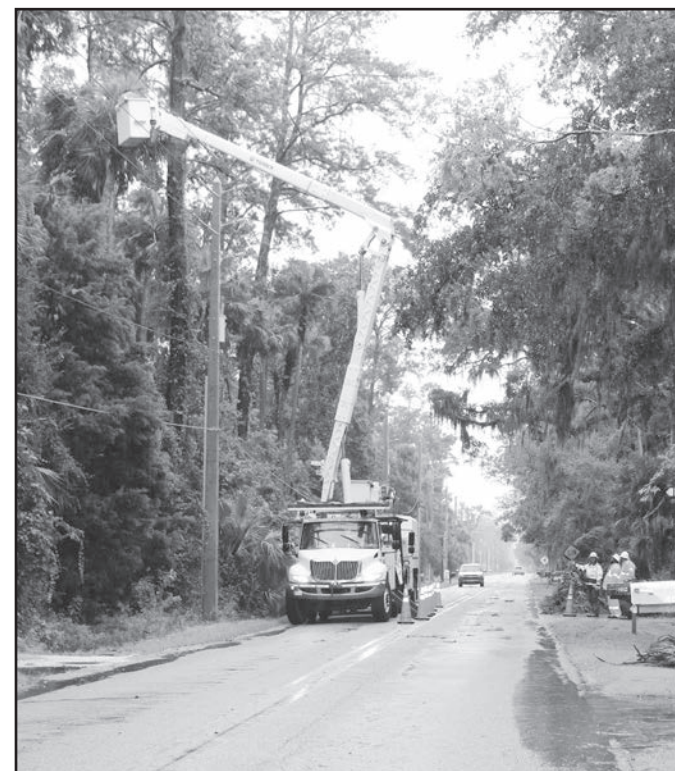
Power crews work to restore service along Roscoe Boulevard. Photos by Susan Griffin
