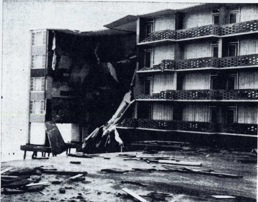
THE SEA IS CRUEL — This is the Atlantic Sands Motel at Rehoboth Beach after the cruel seas of Tuesday and yesterday finished clobbering it. The boardwalk edifice is only
