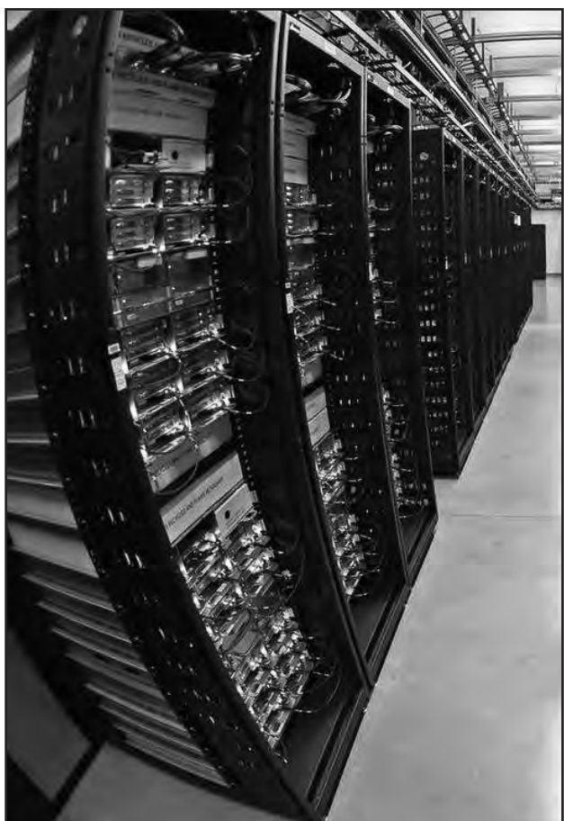
Rows of servers fill Data Hall B at Facebook's Fort Worth Data Center. A Dallas company plans a data center near Benbrook, Texas.
