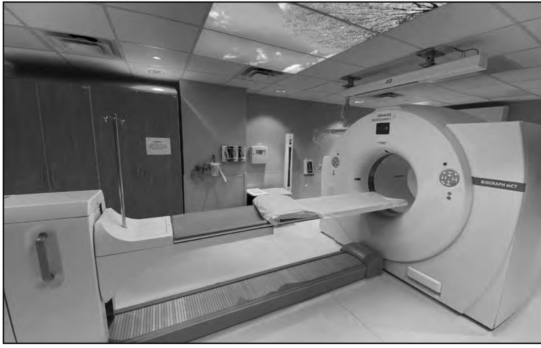
Imaging equipment installed at Guthrie Cortland Medical Center is among improvements in services at the facility in recent years.
