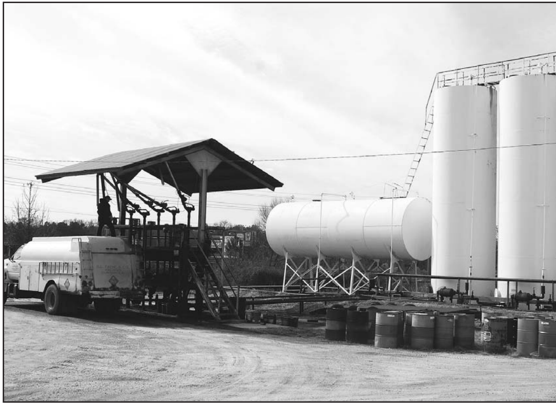
Power supply: These tanks behind the H.D. Payne store can hold up to 2,000 gallons each of fuel oil, kerosene or diesel. Gas products make up one of the top sellers for the old-fashioned hardware store, which has been in business since 1932. — Photo by Bristow Marchant
