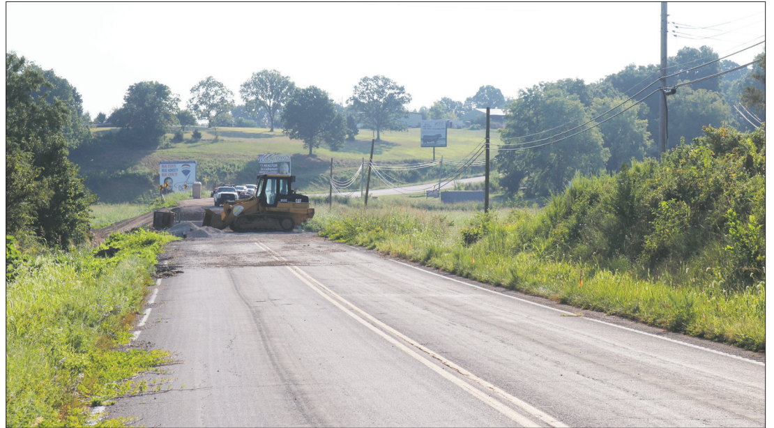
Work continues on the Goodwin Hollow Creek Bridge on Route 64. Visitors to Bennett Spring are directed to take Route 32 to Route OO.
